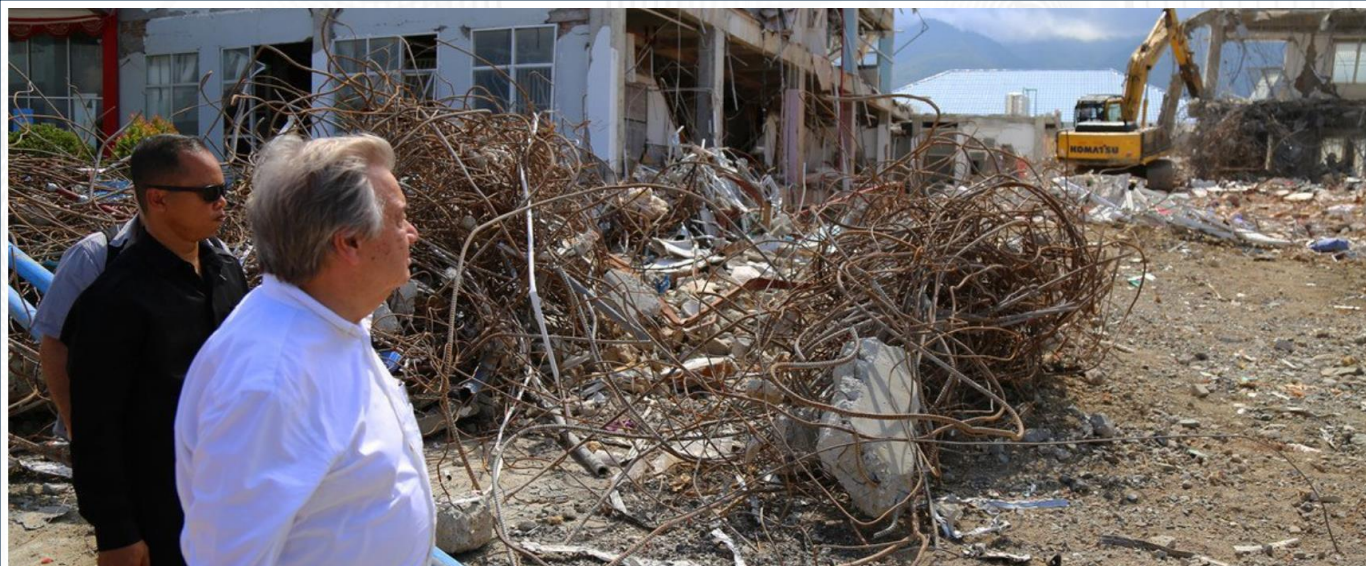
OCHA/Anthony Burke | The UN Secretary-General António Guterres inspects damage to Anutapura public hospital, in Palu on the Indonesian island of Sulawesi, following an earthquake and tsunami in September. (12 October 2018)
